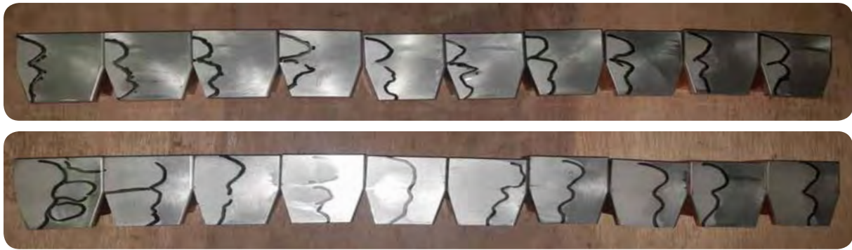
Figure 2- Pattern of damaged areas on babbitt surface of main thrust pads in gas turbine Urmia-3 detected during the second emergency repair
