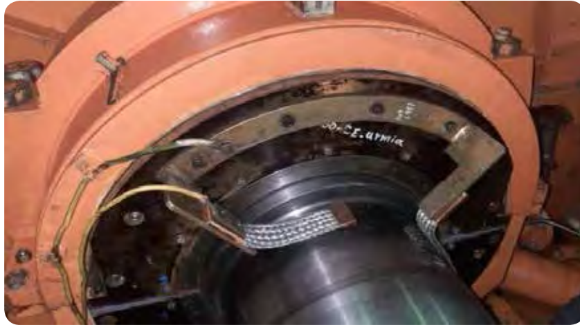
Figure 5- Contact of flexible copper braids with rotor of a generator for discharging stray currents
