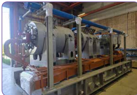
Figure 6- The First High-Pressure Gas Storage Compressor Unit after Packaging in TUGA
